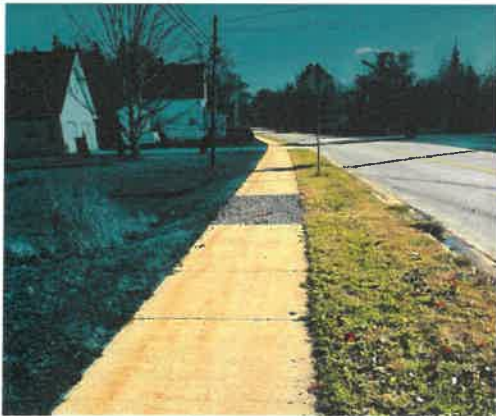
Gravel patch in between concrete paving
