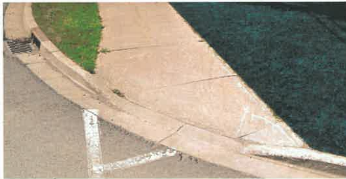
Curb ramp wider than the curb edge
