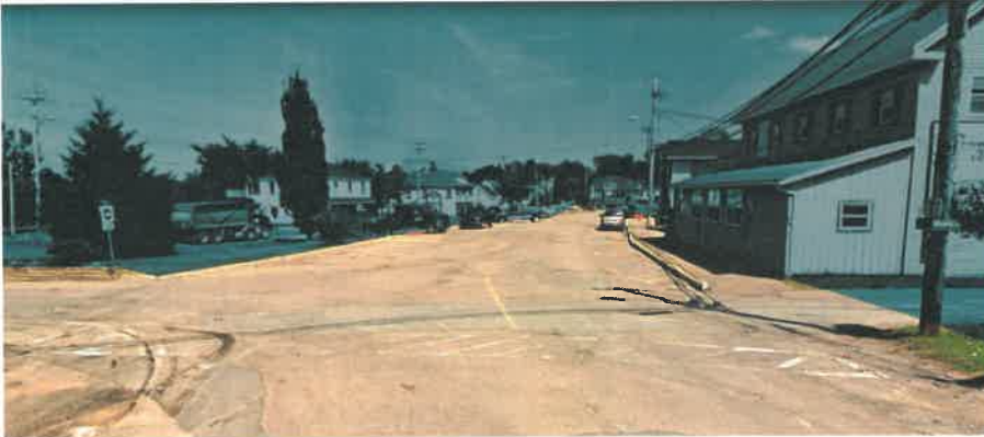
Crosswalk with faded marking and no signage
